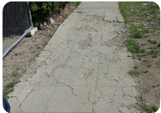
Figure 9 – Sidewalk Segment Rated as Poor
