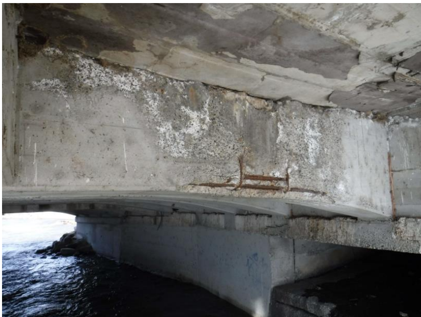
Figure 2. North Bridge (Number B1532), Spalling and Exposed Rebar
