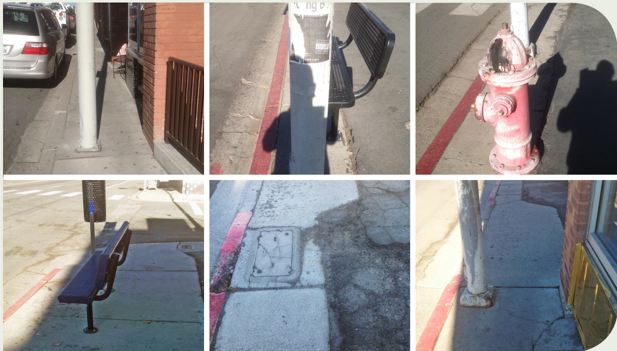
Figure 4.4 - Sidewalk deficiencies (pictures courtesy of Barry O'Sullivan)
